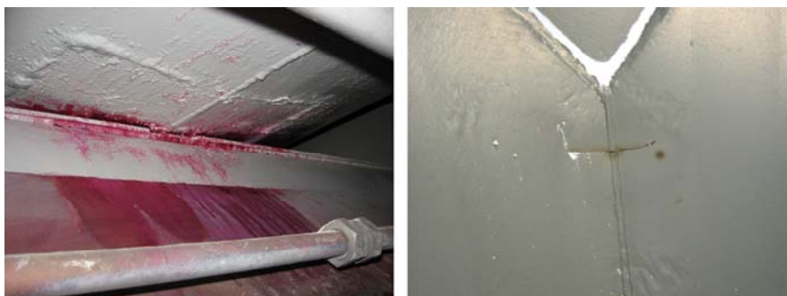
Sl.2 Observed cracks on the construction
